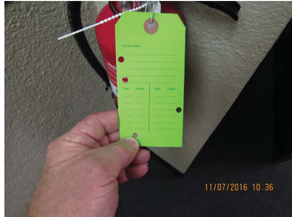
Exhibit 4-16 Hand-Held Fire Extinguisher at ISOK/OVCA has Not Received Its Monthly Inspection
