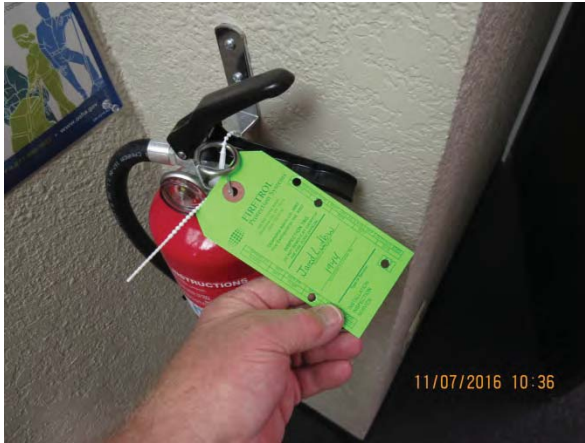
Exhibit 4-15 Hand-Held Fire Extinguisher at ISOK/OVCA has Not Received Its Yearly Inspection
